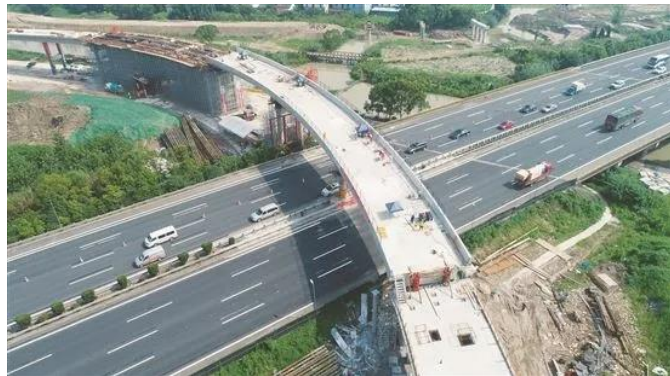
落梁整体航拍图
